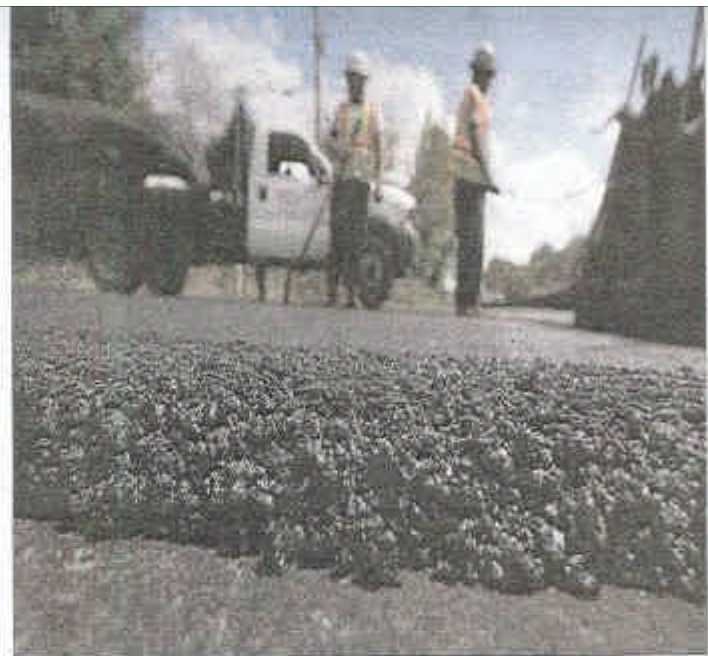
Lojac workers pave Old Hillsboro Road with a warm mix. The asphalt, which is about 100 degrees cooler than traditional hot mix, is much easier on workers laying it.
