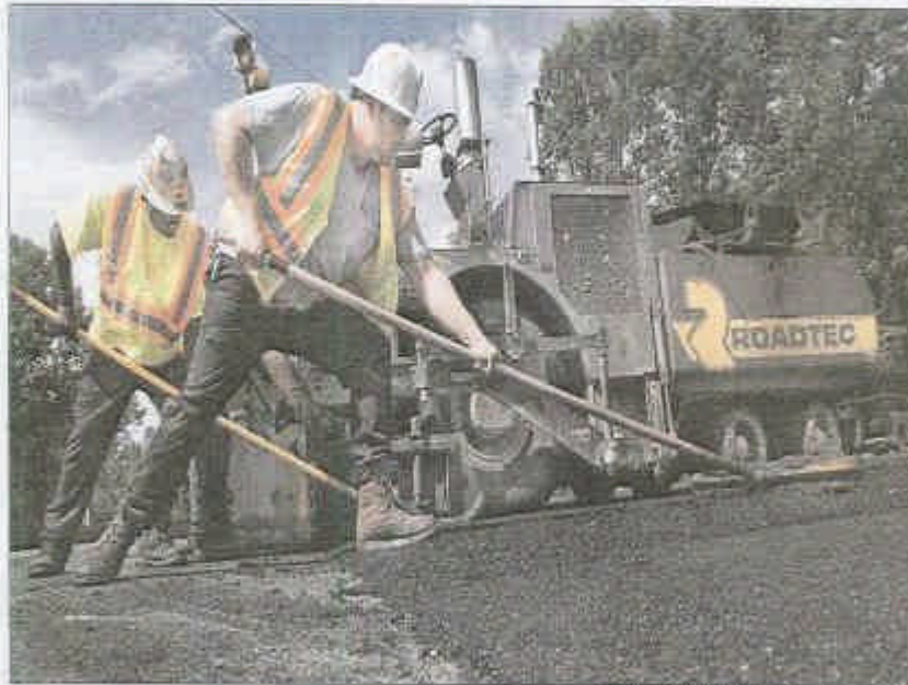
PHOTOS BY GEORGE WALKER IV / THE TENNESSEAN Lojac Enterprises workers Brian Phillips, left, and Josh Buck spread warm-mix asphalt on Old Hillsboro Road in Williamson County. The company and Tennessee Department of Transportation will test the cleaner, less harmful mix.
